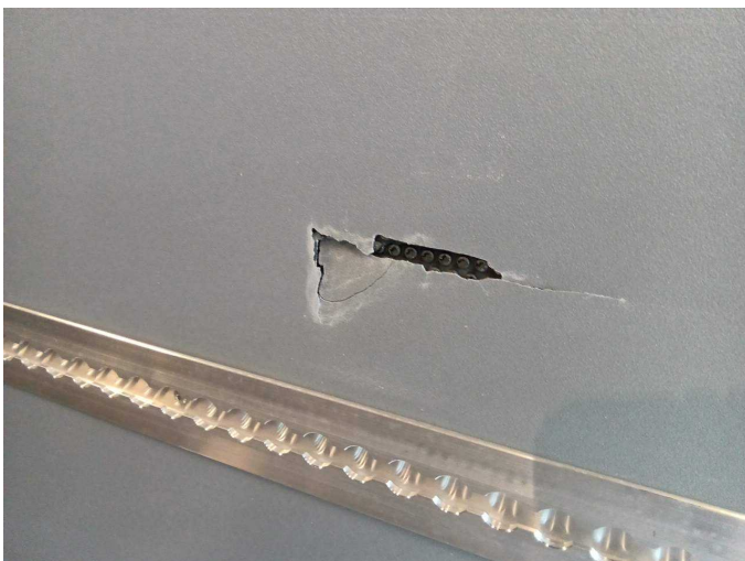
Damage 9: Trim / covers: Cargo area - lining - right side (Mitte) - Broken / torn - Replace
