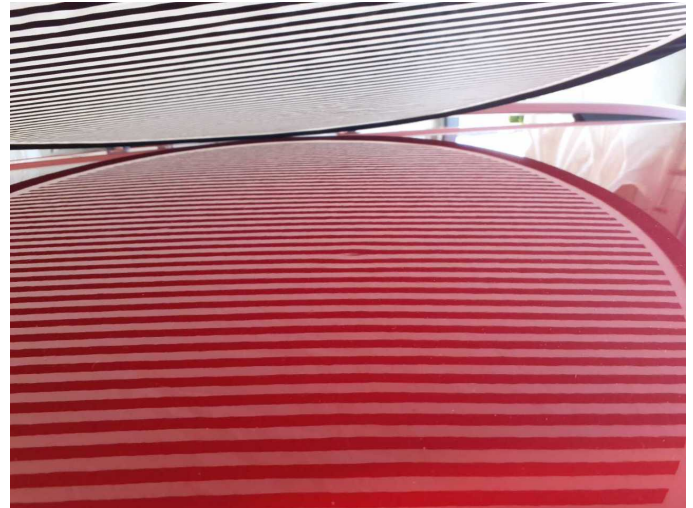
Damage 3: Roof: Roof - dent(s) - Smooth repair work
