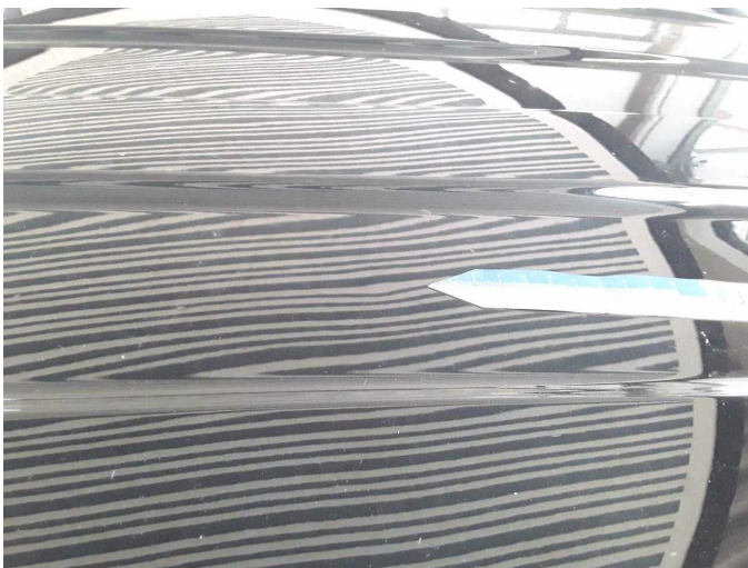
Damage 6: Roof: Roof - dent(s) - Smooth repair work
