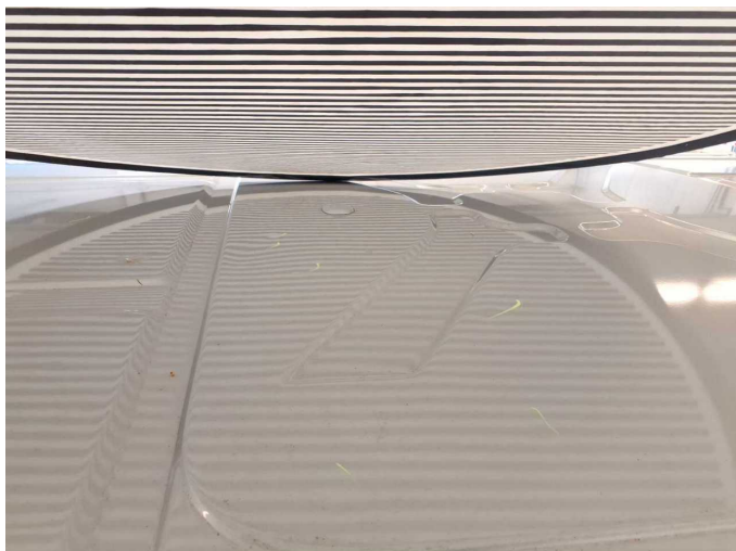
Damage 12: Roof: Roof (Dellen+ Verformung) - Deformed - repair according to calculation
