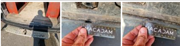
Rear bulkhead lining, Broken, Replace
