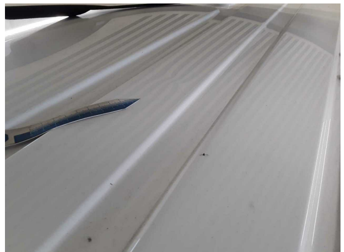
Damage 3: Roof: Roof - dent(s) - Smooth repair work
