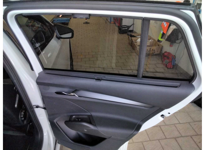
Damage 1: Trim / covers: Door trim - rear right side (Sonnenblenderollo) - Non-operational - Perform diagnosis
