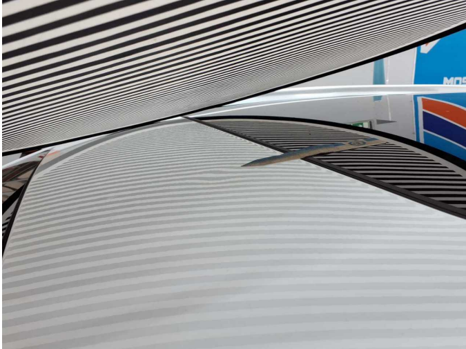
Damage 5: Roof: Roof - dent(s) - Smart repair
