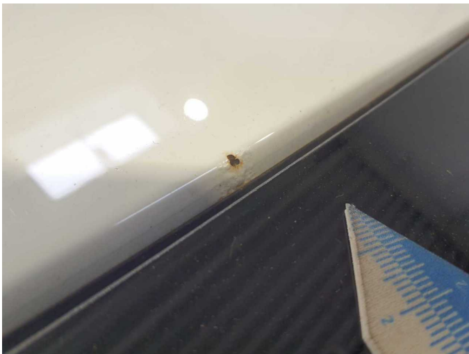
Damage 10: Roof: Roof - Corrosion - Repair and paint
