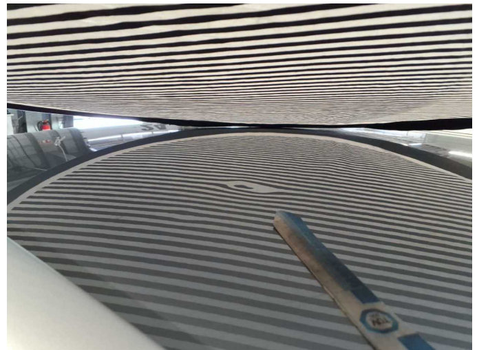
Damage 6: Roof: Roof - dent(s) - Smooth repair work
