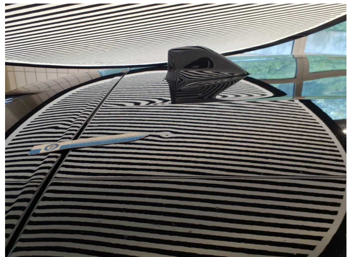
Damage 5: Roof: Roof - dent(s) - Smooth repair work
