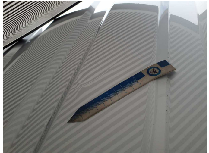
Damage 8: Roof: Roof - Deformed - Repair and paint
