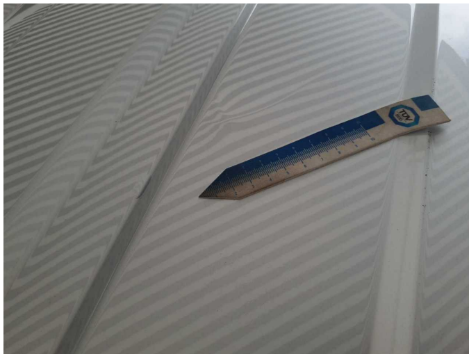
Damage 8: Roof: Roof - Deformed - Repair and paint
