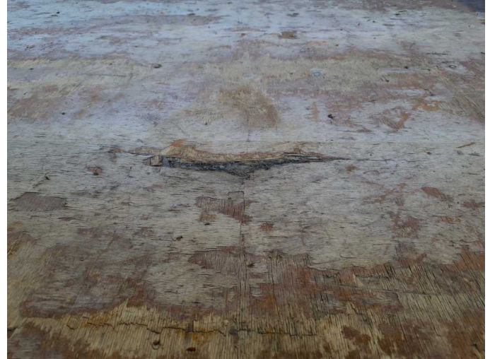
Damage 13: Interior: Cargo area floor - Broken / torn - Loss in value
