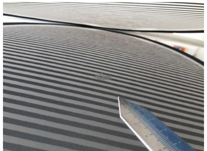
Damage 13: Roof: Roof (Anätzung) - Paint defect - Repair and paint
