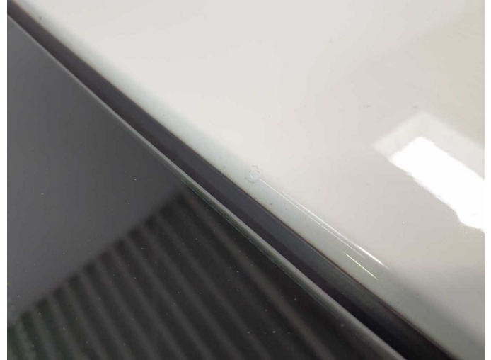
Damage 14: Roof: Roof - Dent / paintcoat damage - Paint
