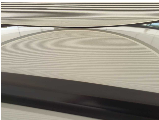
Damage 14: Roof: Roof - Dent / paintcoat damage - Paint
