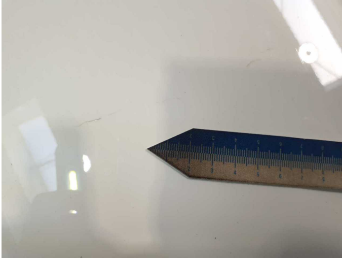
Damage 14: Roof: Roof - Dent / paintcoat damage - Paint
