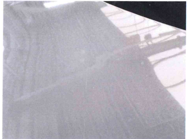
Unfall 1: Dach, Front
