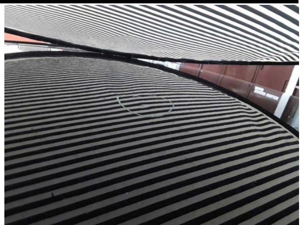
Damage #5: Roof: Roof - dent(s) - Smooth repair work
