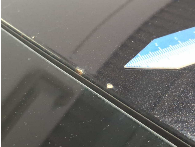
Damage 9: Roof: Roof - Corrosion - Paint
