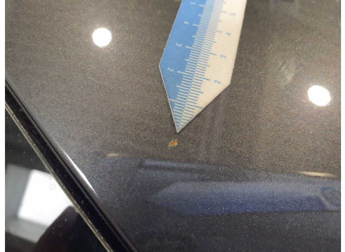
Damage 11: Roof: Roof - Corrosion - Repair and paint
