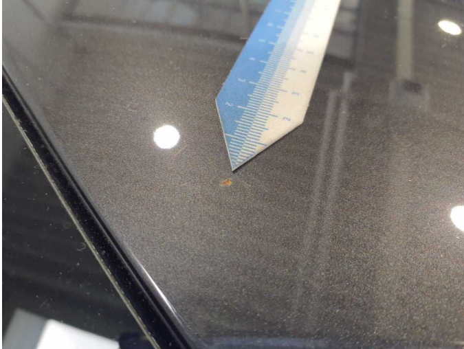
Damage 11: Roof: Roof - Corrosion - Repair and paint
