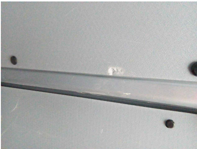
Damage 4: Sliding door, right: Trim - Holes - Replace
