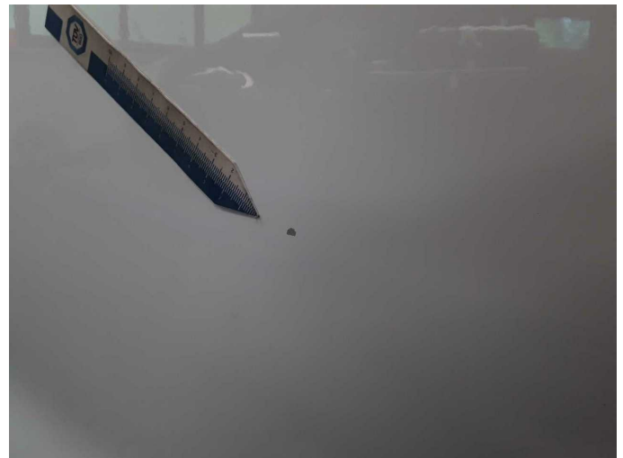
Wear and tear 1: Sliding door - left side: Sliding door - Stone chips - No deduction
