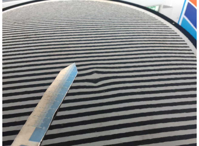
Damage 5: Roof: Roof - dent(s) - Smooth repair work
