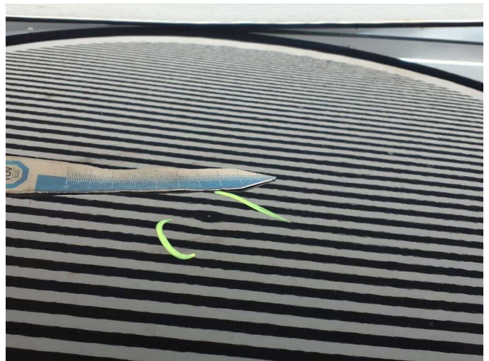
Damage 5: Roof: Roof - dent(s) - Smooth repair work
