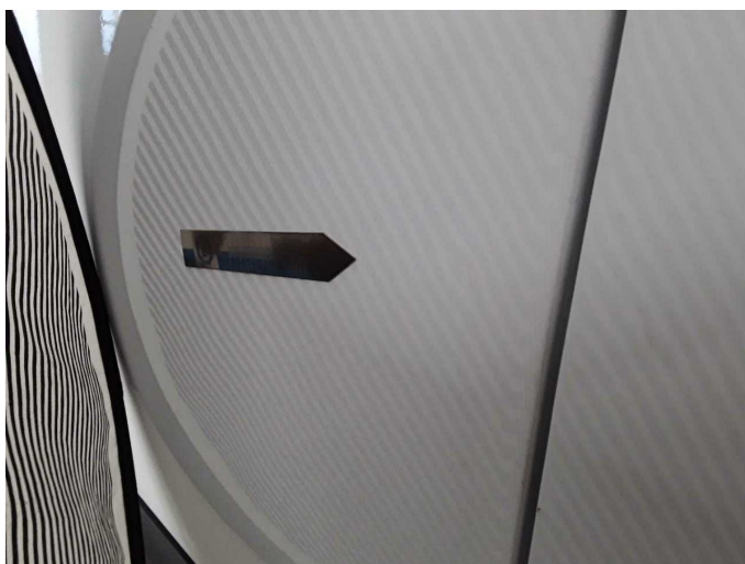
Wear and tear 1: Sliding door, right: Sliding door - dent(s) - No deduction
