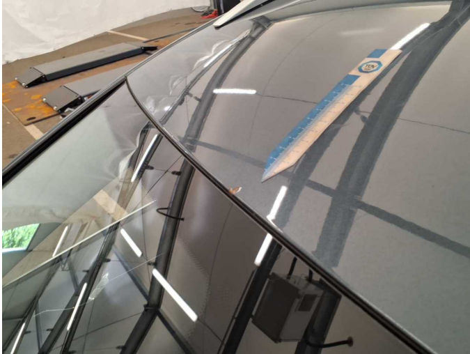
Damage 10: Roof: Roof - Corrosion - Repair and paint
